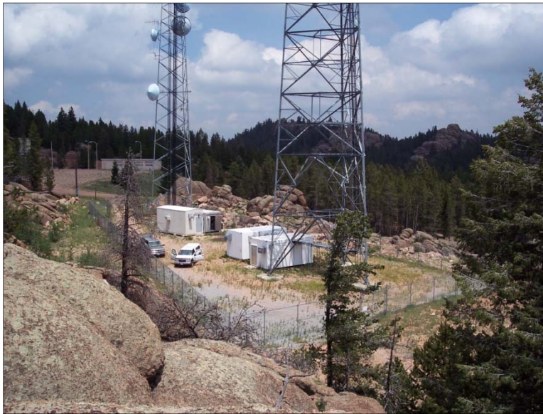
Photo 3-20. West Creek Repeater
