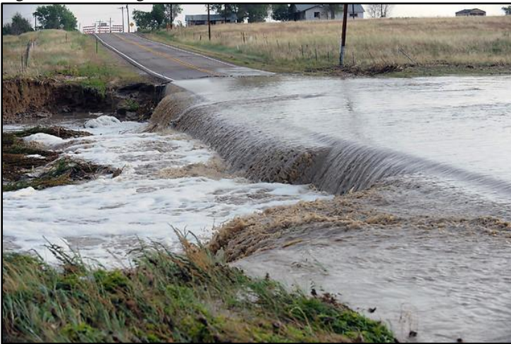
Figure 2: Flooding in Aurora on 6/6/12.
