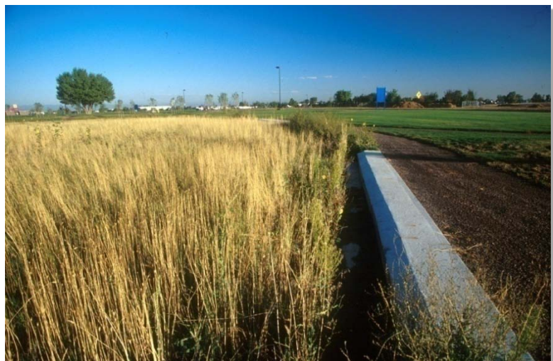
Photograph GB-2. This level spreader carries concentrated flows into a slotted pipe encased in concrete to distribute flows evenly to the grass buffer shown left in the photo. Photo courtesy of Bill Wenk.
