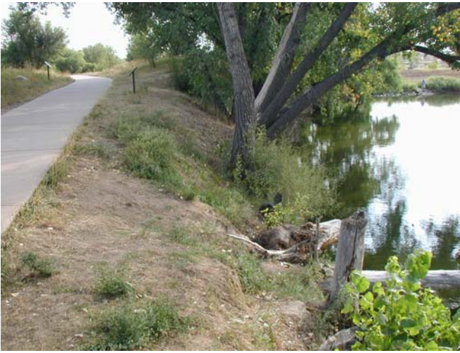
Overland Pond – Before. Note vertical bank erosion threatening mature trees and trail.
