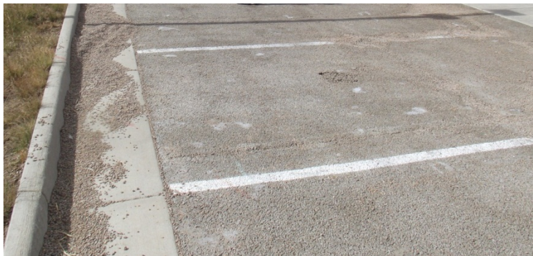
Golden, CO: The National Renewable Energy Laboratory's pervious concrete demonstration pad two years after construction. Note the large quantity of concrete surface aggregate in the gutter section.
